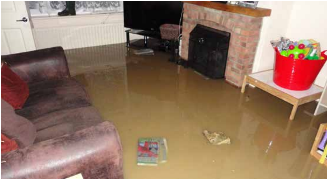
Local Flooded House
